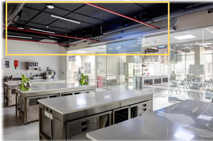
Figure (19): Kitchen zones where the exposed ceiling is existing which includes all the required facilities (Lighting, air-condition, fire alarms and firefighting systems ...)
