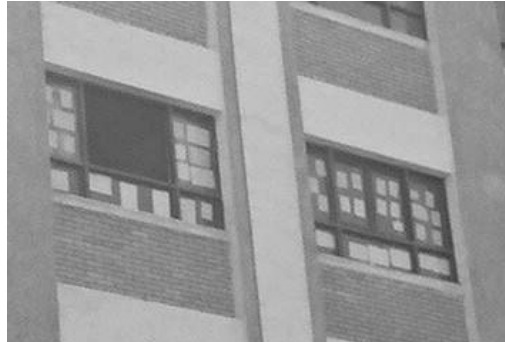
Figure 7: Windows covered and painted by the occupants after Gado and Mohamed (Gado et al. 2005)
